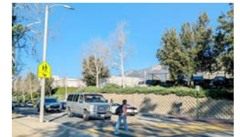
Missing pedestrian curb ramp at a high-visibility crosswalk. ↴ Los Osos High School
