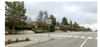
Multi-lane roadway crossing missing pedestrian curb ramps . ↴ John L. Golden Elementary School
