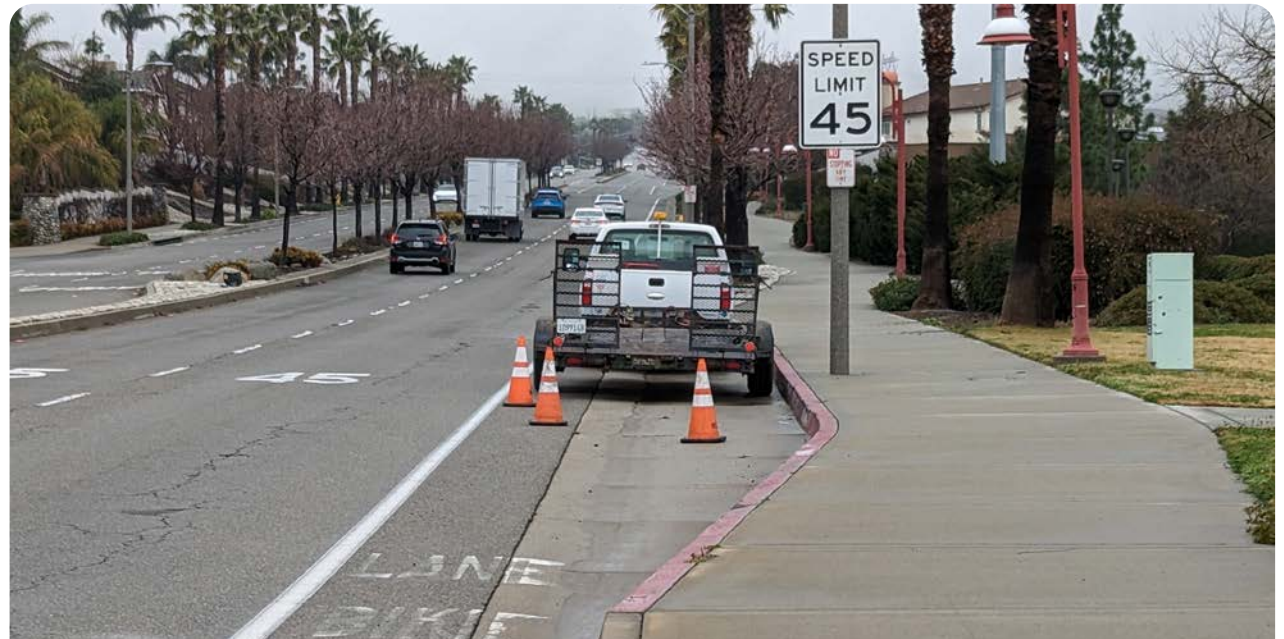
Buffered bike lanes along Day Creek Blvd. can provide a more comfortable bike facility by allowing more space between the bicycle lane and vehicle travel lanes.
