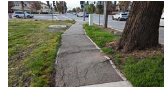
Sidewalk near elementary school buckling due to adjacent tree roots . ↴ Grapeland Elementary School
