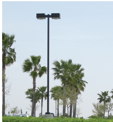
Parking Lot Light
